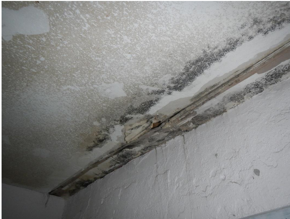
Water damage is pervasive throughout her house Mold is a real health treat for many residents with leaky roofs.
