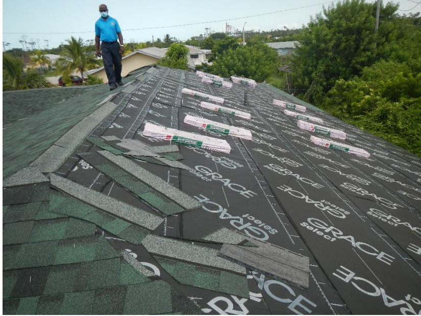
Still leaks-only half a job done
